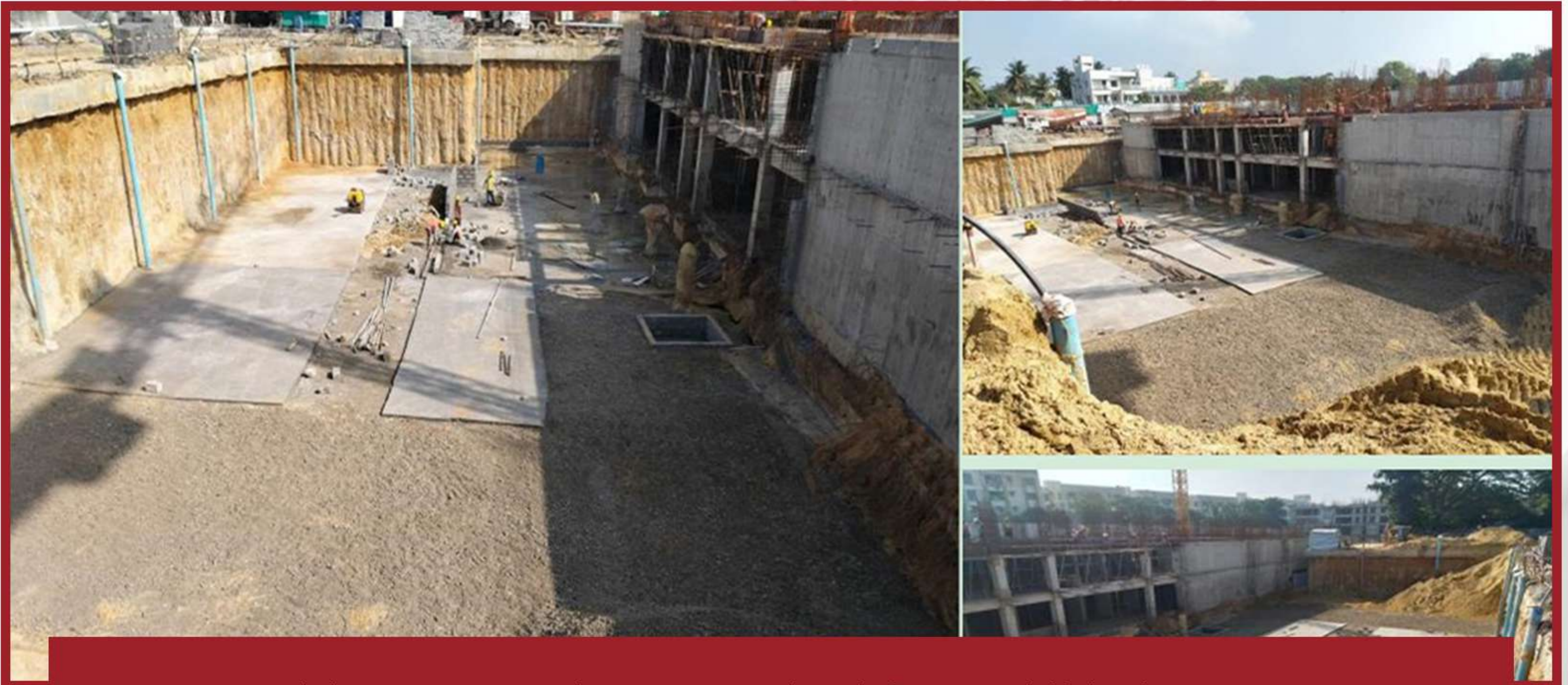
Block C – DEEP excavation works are nearing to complete and raft-pcc & STP Side block works in progress.
