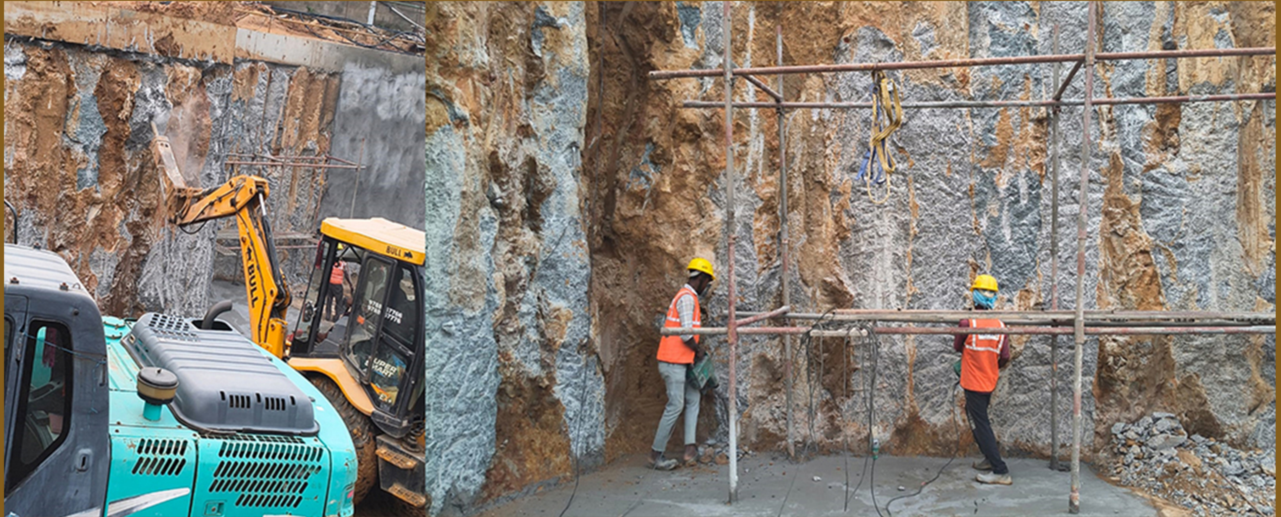
Block B pile bulging concrete Chipping
